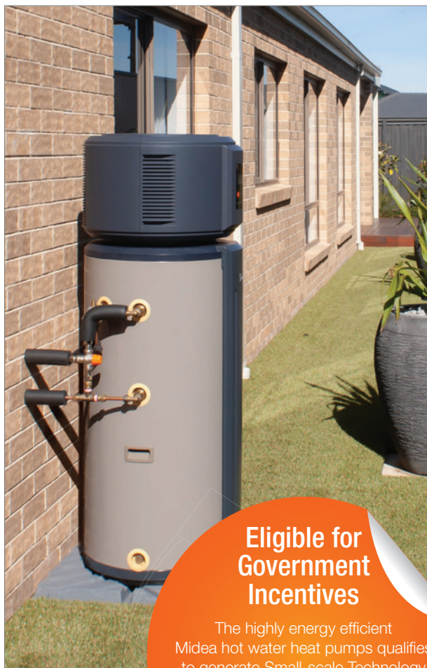
170L Installed Unit
